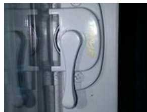
Example of improperly engaged lock: The locking mechanism is in the fully locked position but not engaged. It is closed over top of the outer window lock receiver.
