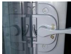
Example of improperly engaged lock: The locking mechanism is half-turned in the locking position, but not engaged with the other half of the window.
