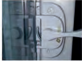
Example of improperly engaged lock: The locking mechanism is half-turned in the locking position, but not engaged with the other half of the window.
