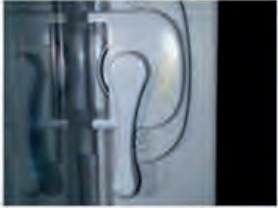
Example of improperly engaged lock: The locking mechanism is in the fully locked position but not engaged. It is closed over top of the outer window lock receiver.
